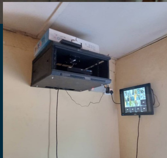
Centralised CCTV for facility monitoring
